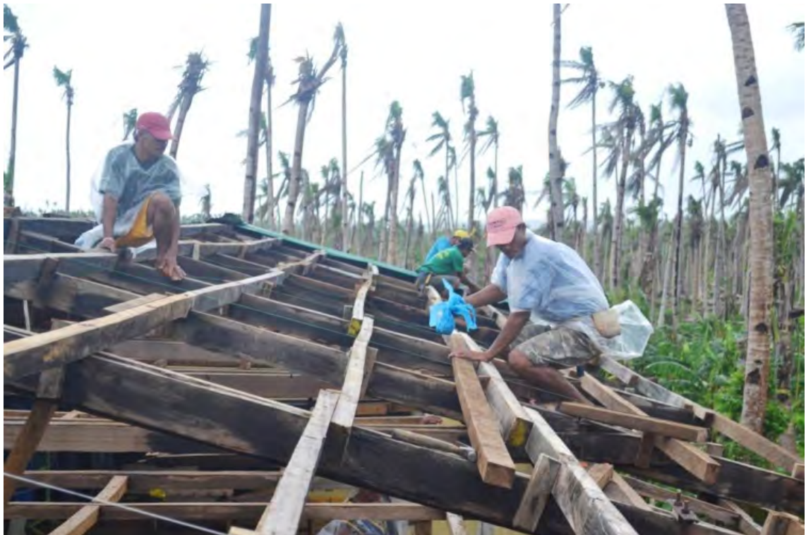
Artisans mounting purlins on the roof of building 12. In 4 days, classes can resume in the 3 classrooms once the GI sheets and ceiling panels are done.
